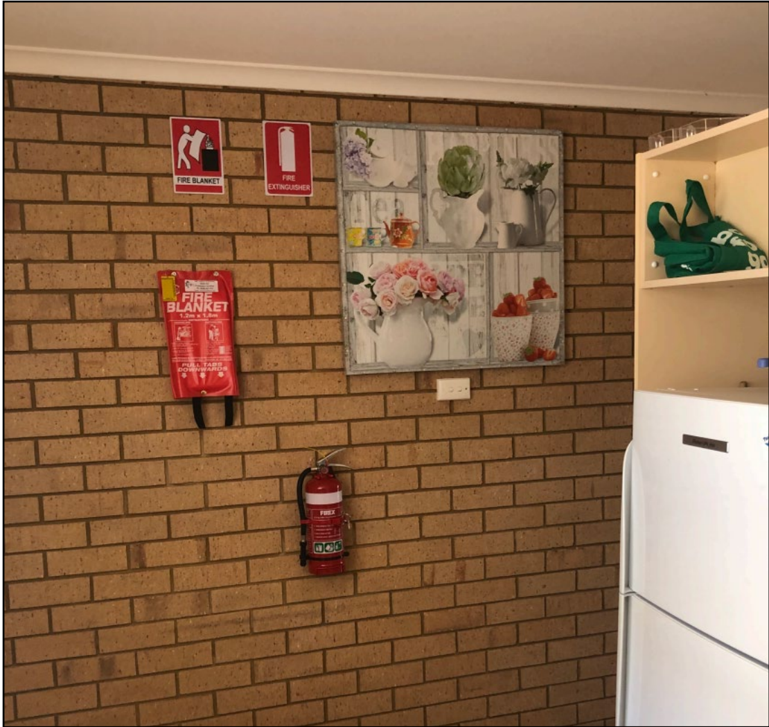
Above: Fire Blanket and Fire Extinguisher
