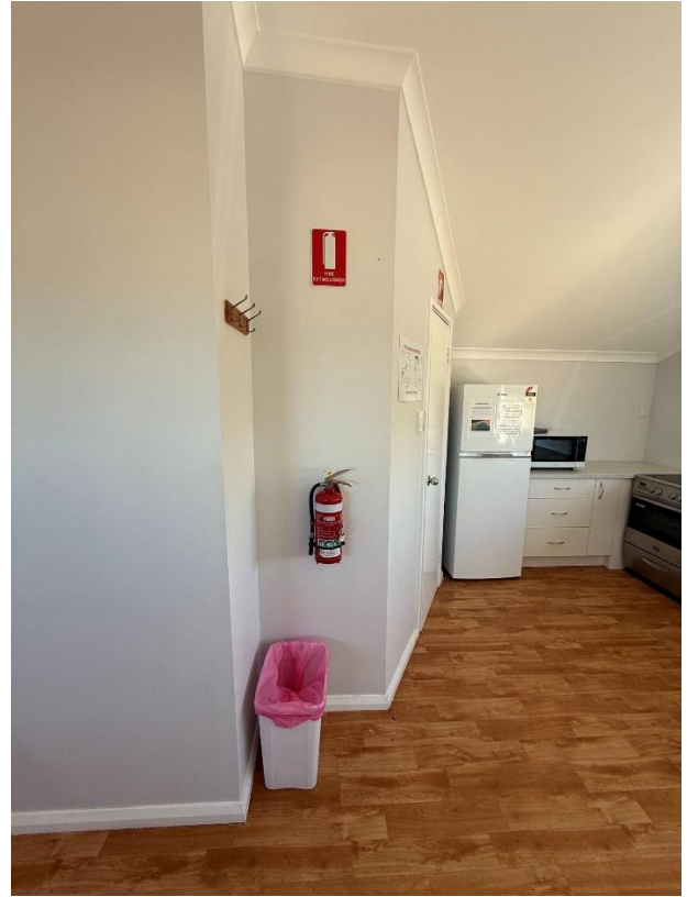
Fire Extinguisher (upstairs)
