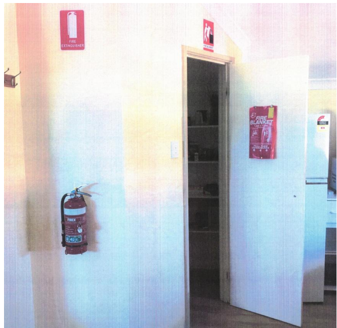
Upstairs Fire Extinguisher & Fire Blanket
