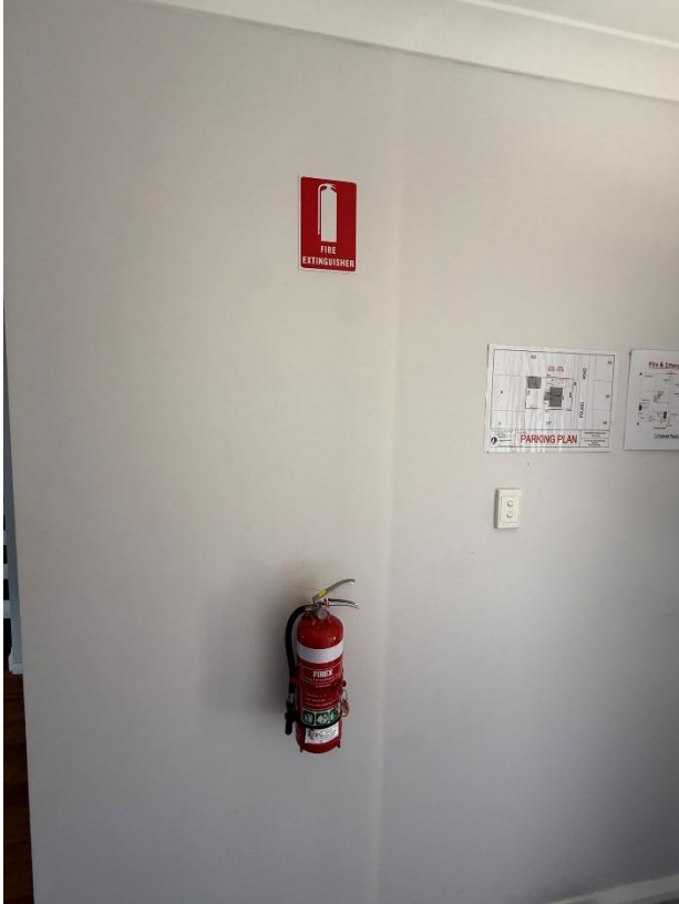
Fire Extinguisher (downstairs)
