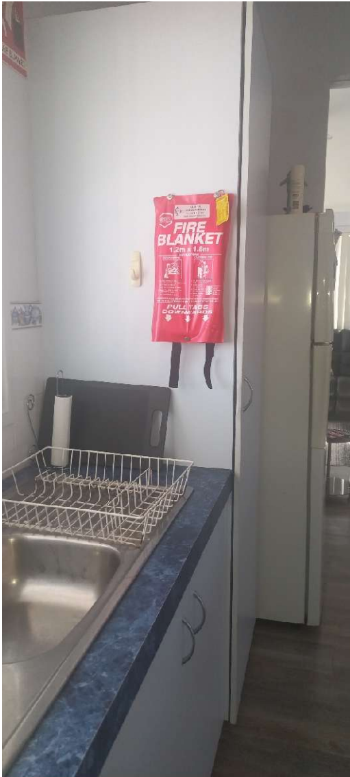
Fire blanket installed
